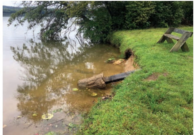
A section of Yellow Creek State Park, Indiana County, before the shoreline restoration project completion.
